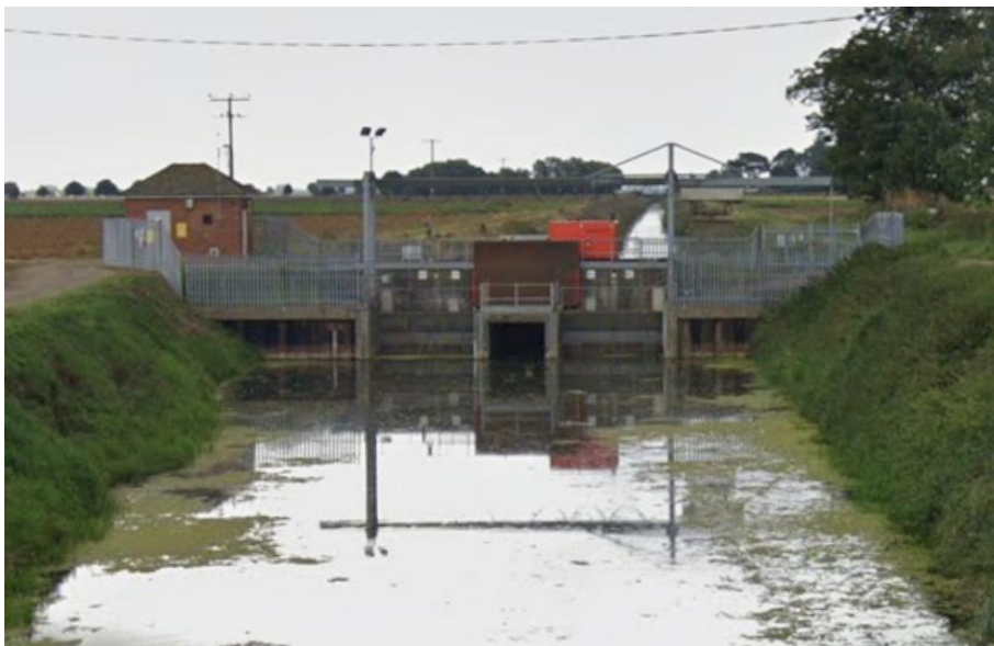
Figure 7 – Street View Image of Wiseman's Pumping Station Sluice, taken from Google Street View 10 .
